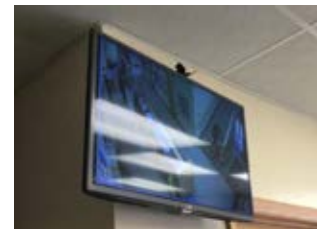
CCTV Monitor in Office
