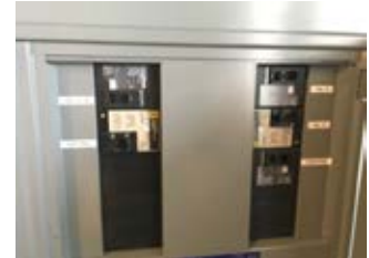
Main Electric Service
