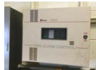
Fire Alarm Control Panel
