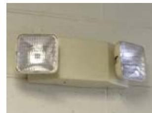
Emergency Lighting Unit
